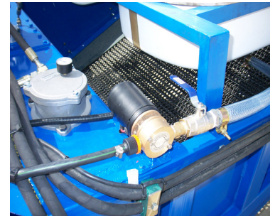
Electric motor of the pump
